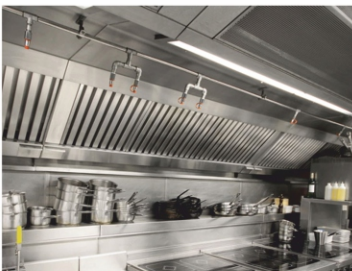
Kitchen Fume Extraction Ventilation System
