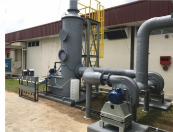
Acid Fume Extraction System
