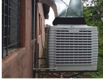
Evaporative Cooling System
