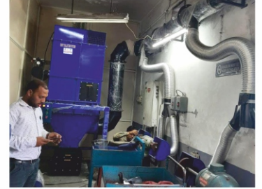
Dust Extraction System
